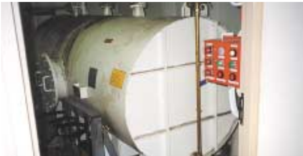
High-expansion foam fire extinguishing system on board
