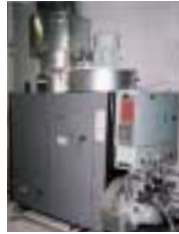
Waste oil incinerator
