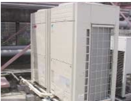
External unit for air-cooled air conditioner installed on the rooftop of our head office.
