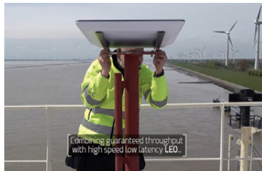
Onboard Starlink installation
