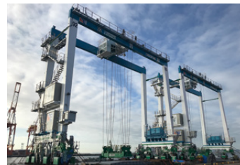
Image of “Near Zero Emission” Transtainer ® , installed at the Kobe International Container Terminal and the Minami Honmoku Pier Container Terminal in Yokohama Port (Photo : Minami Honmoku Pier in Yokohama Port)
