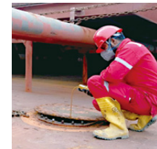
Gas detection in a tank before work
